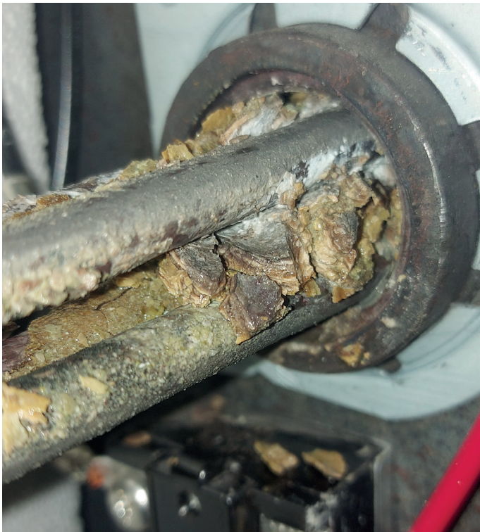
Limescale formation on electric immersion element deployed for primary water heating
