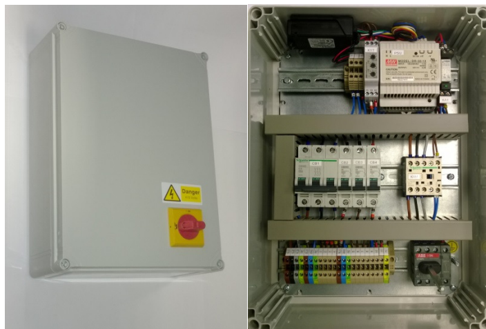
Photo example of the SGE Control Panel EB0025 The ITE Control Panel EB0028 looks similar
